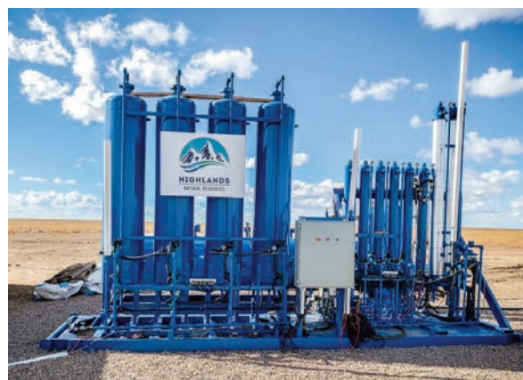
Pressure Swing Absorption Unit – Nitrogen Hydrogen Project in Kansas
